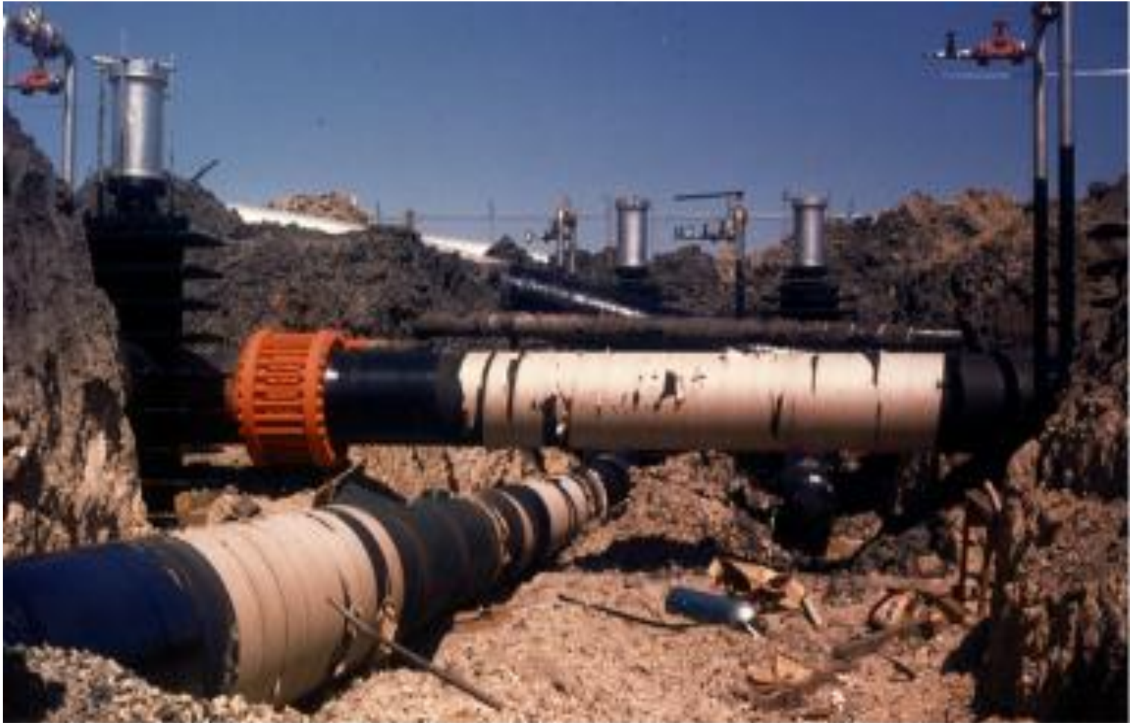
Underground Piping for Station 2 Compressor Station
